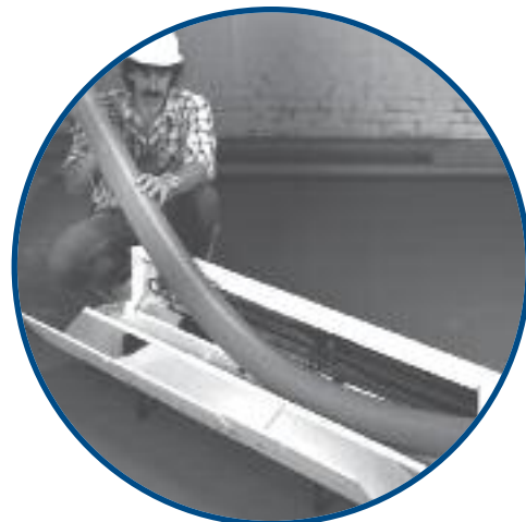
Minimum practice is required to master the three steps in bending nonmetallic conduits and ducts.
