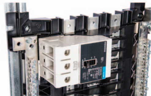
Example of Back-fed xGB Main breaker installed
